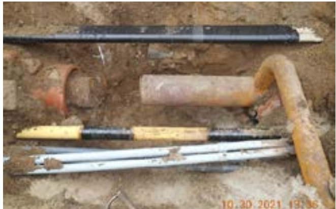
Defective underground piping.
