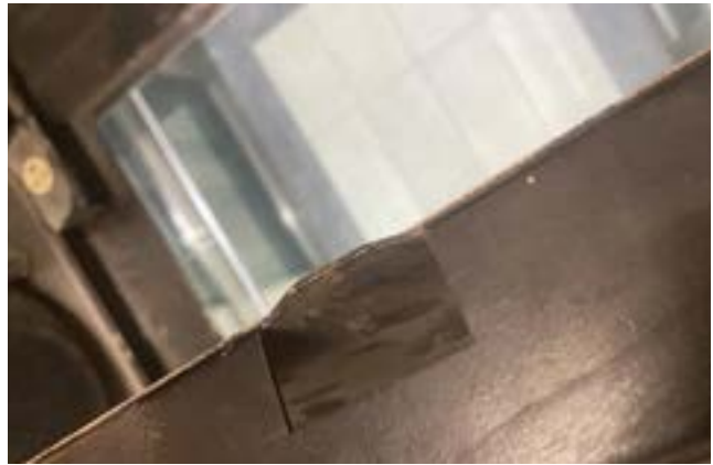
Ceiling hatch pushed hard enough to bend the metal that keeps the door closed.
