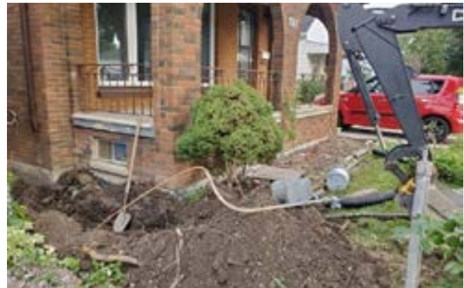
Gas line and meter above ground.
