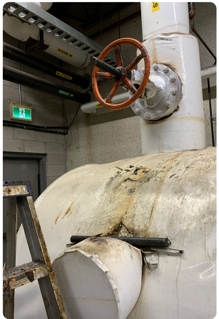
Poorly insulated accumulator steam line
