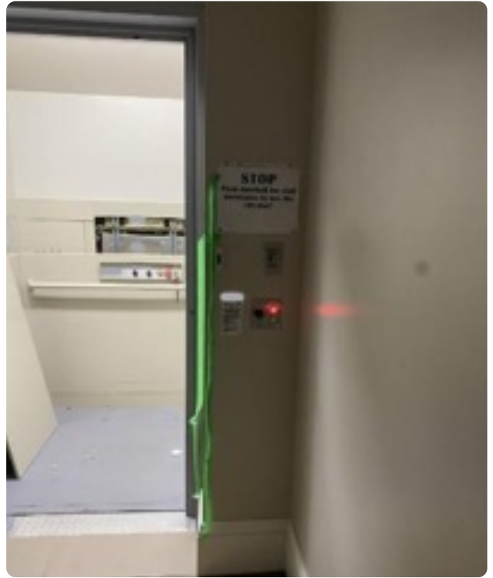
Vertical platform lift interior
