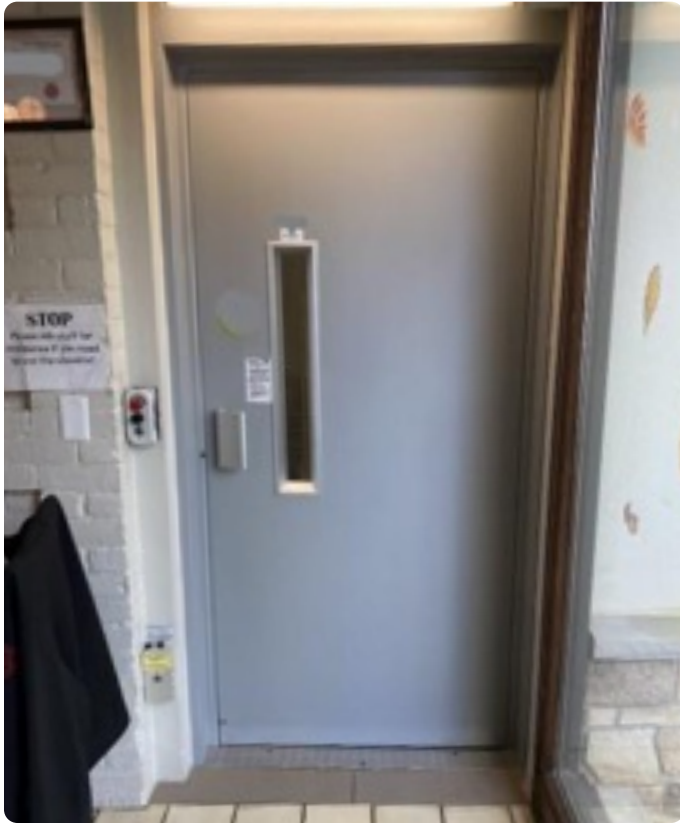
Vertical platform lift exterior
