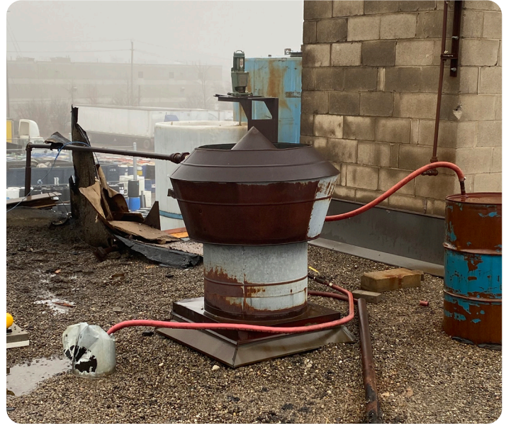
Hoses on rooftop attached to unknown vessel
