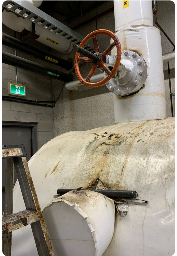
Poorly insulated accumulator steam line
