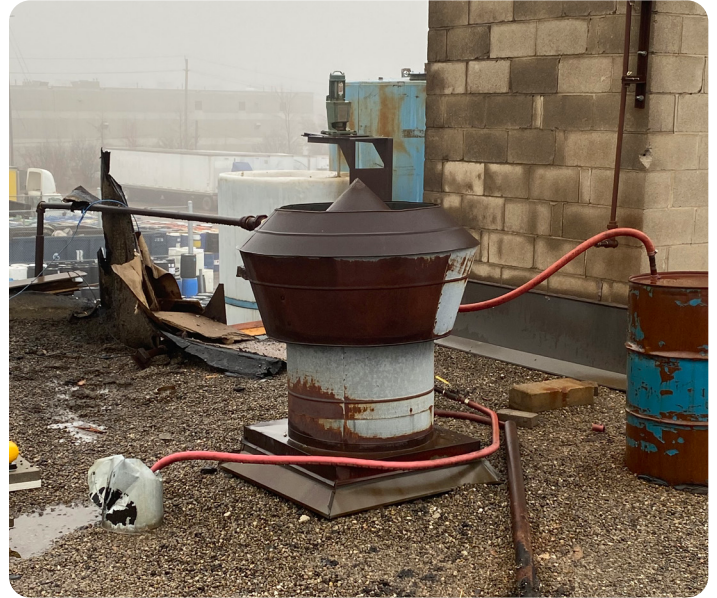
Hoses on rooftop attached to unknown vessel
