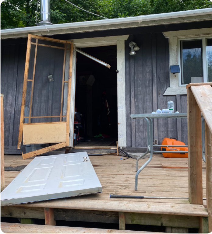
Cottage after explosion
