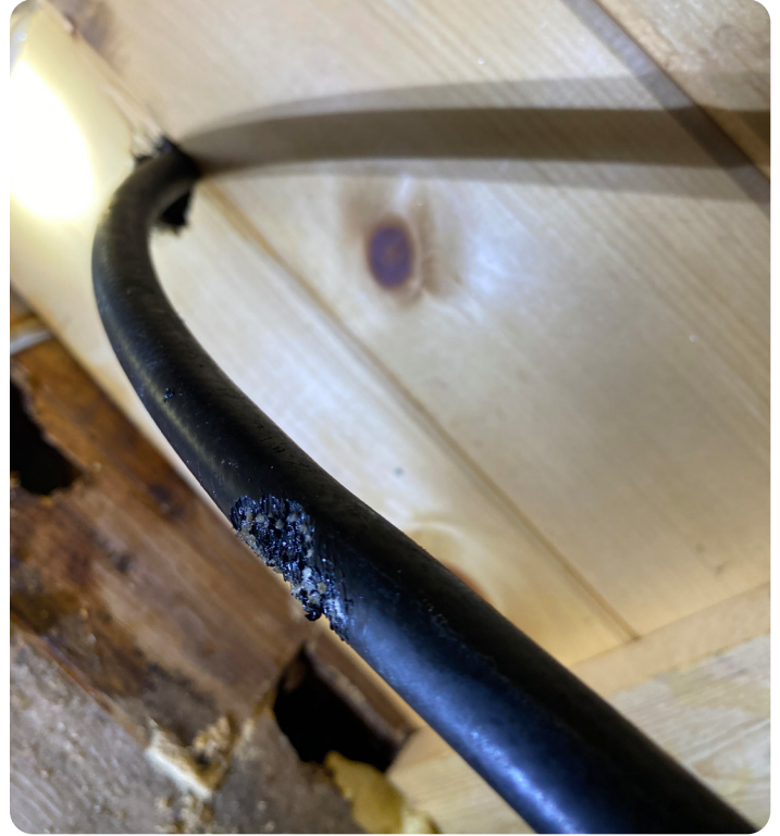
Piping mice chewed through
