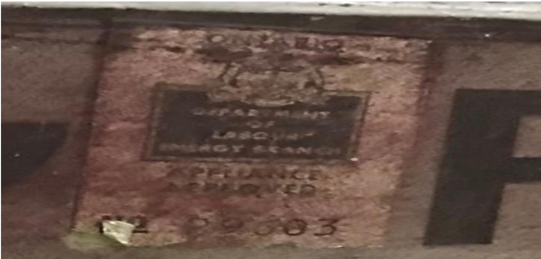
Province of Ontario Department of Labour - Energy Branch Approval Sticker
